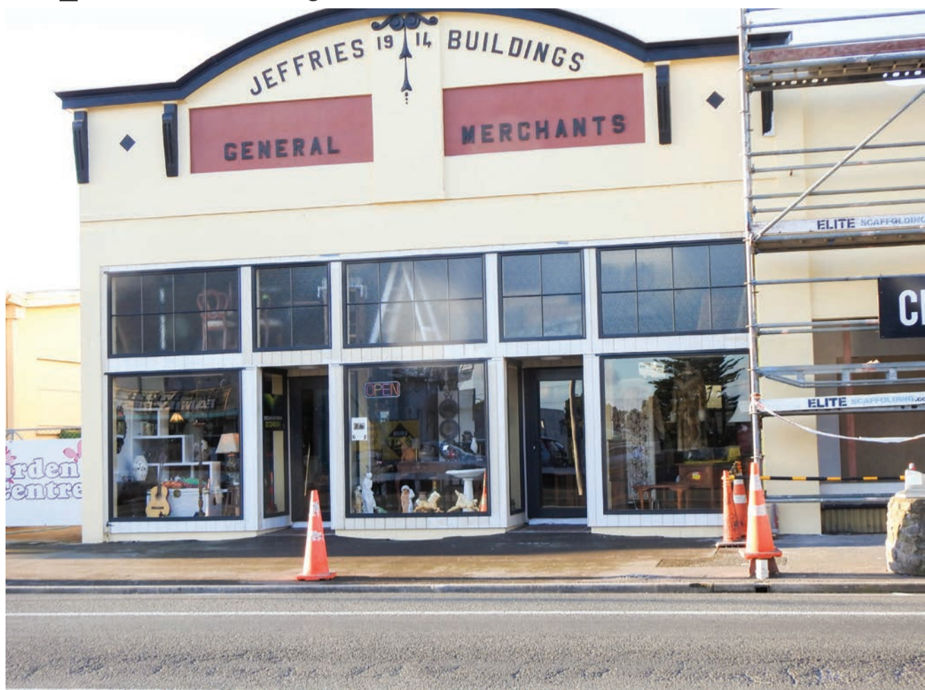
A stunning new façade and windows for one of Opunake's heritage buildings.
